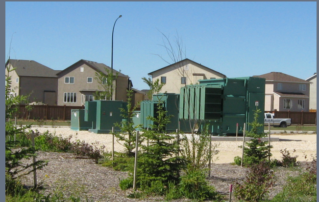
Below: 10MVA, 72kV HVPT Station in a residential setting
